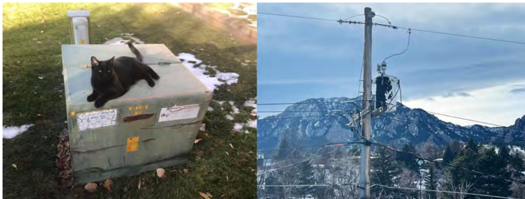
FIG. v Pad-mounted transformer (left), indicating underground distribution lines, and pole-mounted transformer (right), indicating above-ground lines.
